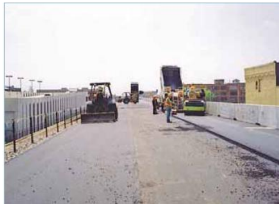
Figure 6. Placing Asphalt Underlayment on the Wichita, KS elevated track section for the mainlines of the BNSF and UP railways
