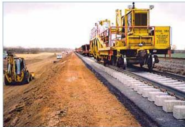
Figure 4. Placing the new track on the BNSF 'transcon' project prior to adding ballast and 'pulling the track up' to achieve the desired ballast thickness
