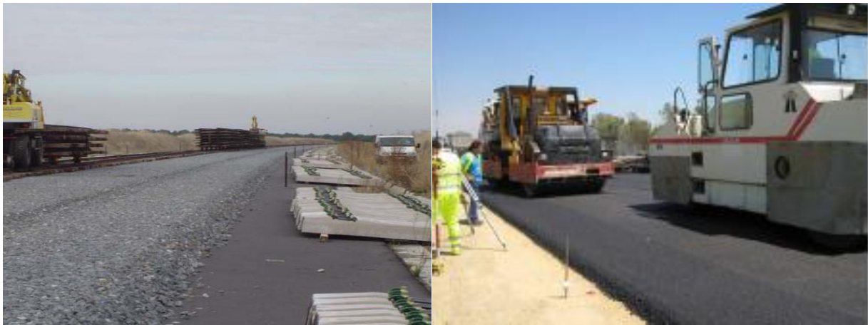
Figure 15. Bituminous subballast sections built on the high-speed line Madrid-Valladolid, section between Segovia and Valdestillas (left) and on the high-speed line Barcelona-French Border, section Sils-Riudellots (right). Source: Teixeira (2009).
